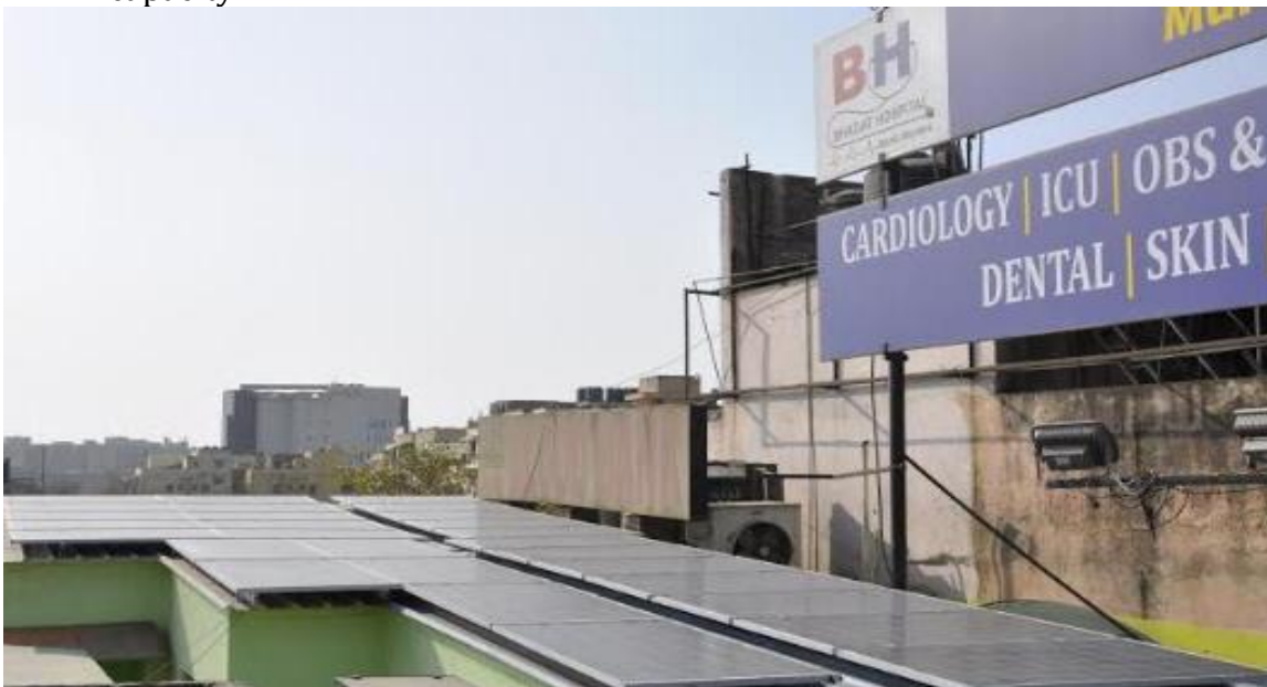
Figure 1: Installed Solar Panel located at the hospital.
