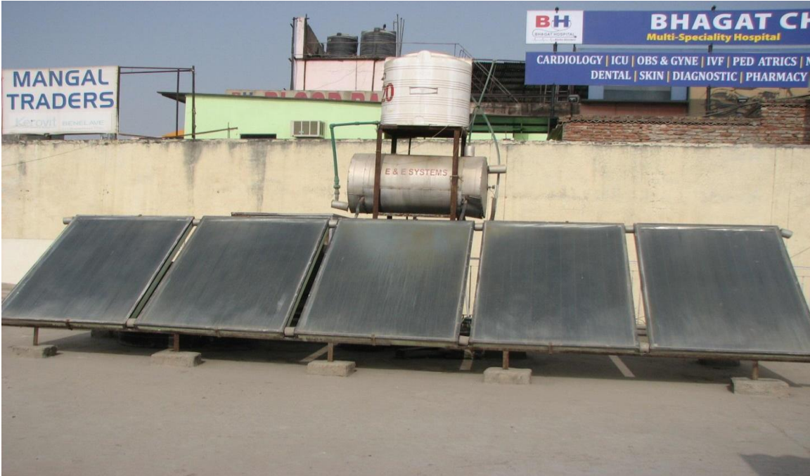
Figure 2: Solar panels used for water heating.
